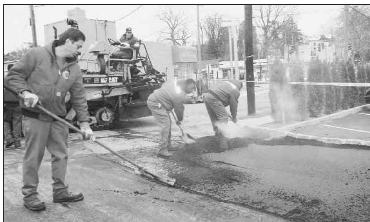
Town of North Hempstead Unit member Bruno Iannelli and other crew members level hot asphalt, with steam rising in several places, before a highway roller goes over the road again.
