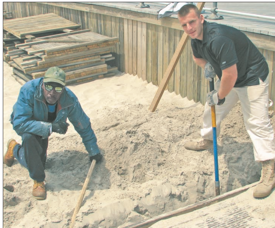
State parks workers Richard Van Horn, left, and Matt Lemonis repair a section of the boardwalk leading to Jones Beach. Parks workers across Long Island have been working to get state, county, town and village parks ready for the summer season after Hurricane Sandy's devastating damage last fall.
