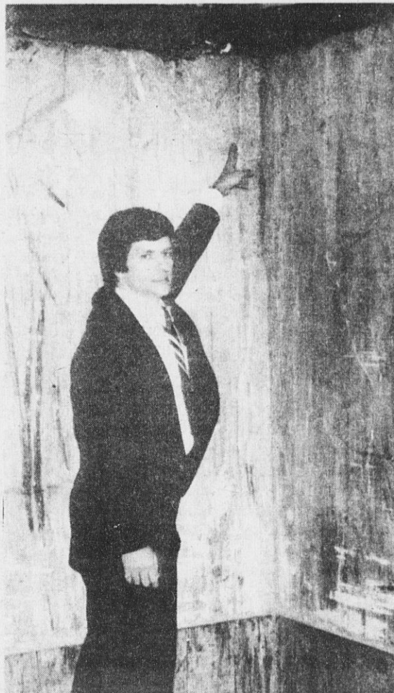
LOCAL 830 Safety Committee Chairman Ralph Spagnolo points to a huge crack in a retaining wall at the Town of Oyster Bay compactor in Bethpage. The Local 830 Safety Committee and CSEA members who work at the facility fear that a truck will back into the wall on the side Spagnolo is standing, the wall will fall and injure or kill someone on the lower level.
