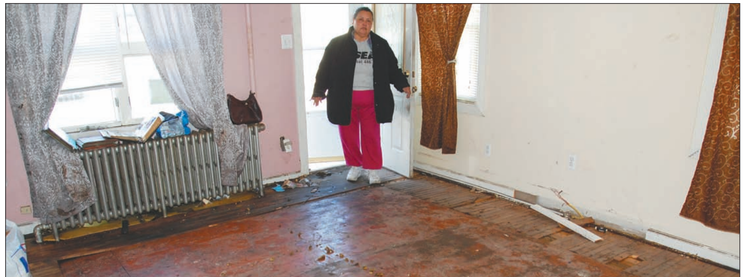
Blanca Maldonado enters her water damaged living room in her Staten Island home.
