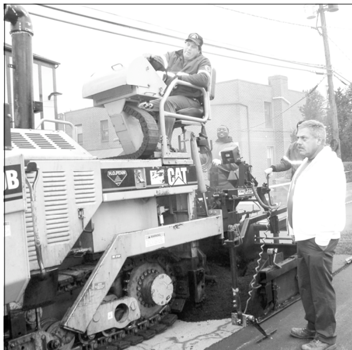
Art Gerhardt, top, and Mike Flaherty, right, are shown while road crew re-paves a road in North Hempstead last winter.
