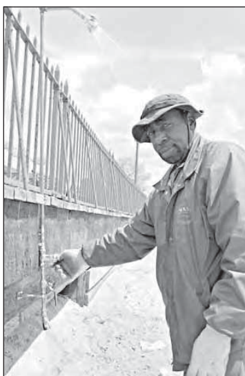
Derrick Graham, a plumber at Playland, makes repairs to an outdoor shower at Playland Beach.
