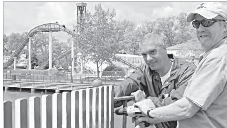
John Fabro, left, and Jim Cody, maintenance mechanics at Playland, prepare to replace fencing at the park. The Log Flume ride is in the background.
