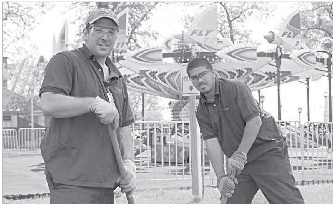
CSEA members Joe Greco, left, an electrician at Playland, and Anthony Fogal, an electrical helper, prepare a vacant site where a ride called the Yo-Yo is slated for installation. In the background is the Kite Flyer ride.
