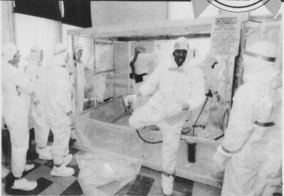
NO SPACE INVADERS but rather a safety-suited crew of Syracuse City School District maintenance workers during an intensive early training session. The men are in the process of hanging plastic sheets on a framework used in classrooms before asbestos removal. (Photo courtesy of Syracuse Newspapers/David Lassman)
