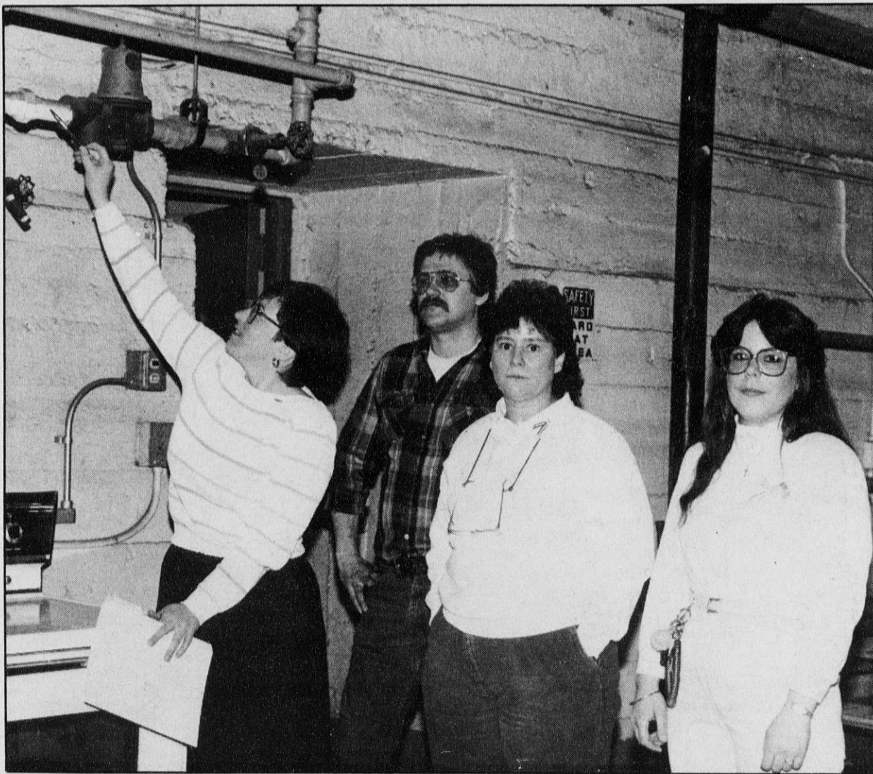
THIS IS IT — CSEA OSH Coordinator Wendy Hord points out asbestos and coal dust on the pipes in the Hudson River Psychiatric Center powerhouse. With her are, from left, Stationary Engineer Michael Gray, Local 410 President Judy Watts and Local 410 Vice President Laura Sleight-Legname.
