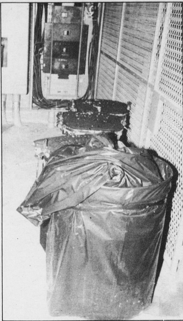
GARBAGE CAN, covered with an unlabeled plastic bag, contains PCB-contaminated soil, caused by transformers such as those line up behind the can.
