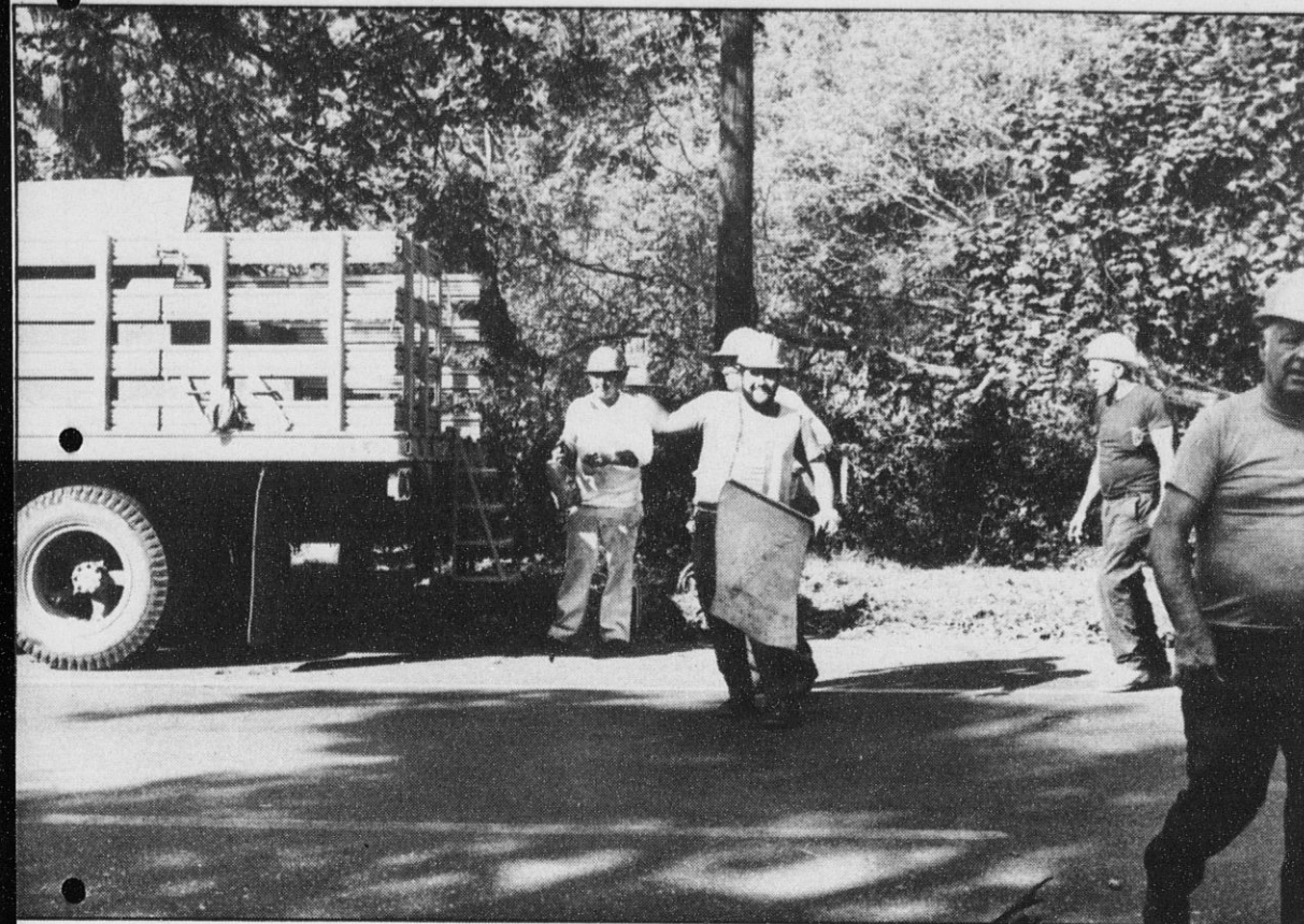
SUMMER MEANS PLENTY OF HIGHWAY REPAIR projects across the state. This crew was at work on a Long Island highway.
