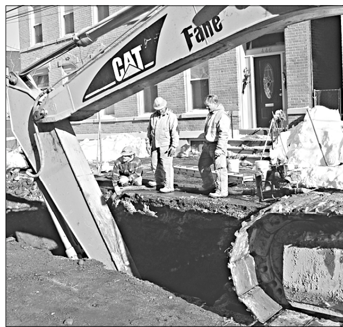
Troy Department of Public Utilities workers brave sub-zero weather to repair a broken water main, one of several that burst recently.
