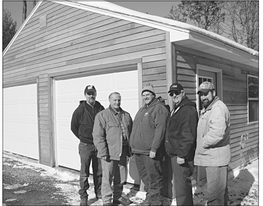
Members of CSEA's Town of Greenport Unit stand in front of the garage they built for the town. From left to right are Mark Gaylord, Roger Rote, Chip Roberts, Dan Kenneally and Unit President Pat Nolan. Other CSEA members who helped build the garage but are not shown are Fred Fuchs, Anthony Porreca and Bob Poulter.
