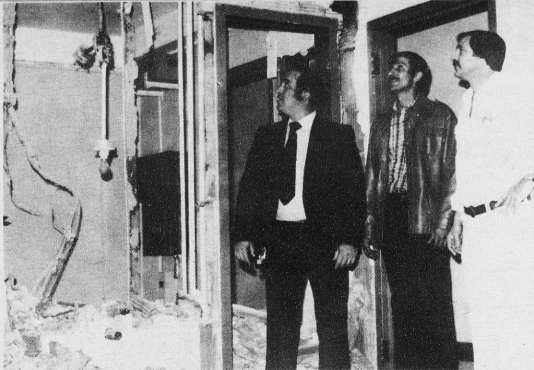
INSPECTING SOME DEMOLITION WORK done as part of the rehabilitation project at Westchester Developmental Center are, left to right, Field Representative Larry Natoli, Local 432 Vice President Lee Rushford and Local 432 President Gary Eldridge.
