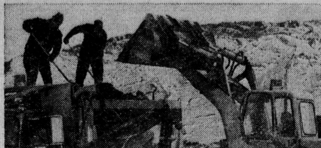
Robert Booth, left, operator, and Howard Fralick, wingman, help get winged State plow ready for the next snowfall as loader digs into mountain of 5,000 yards of sand at one point at Department of Transportation station south of Watertown.
