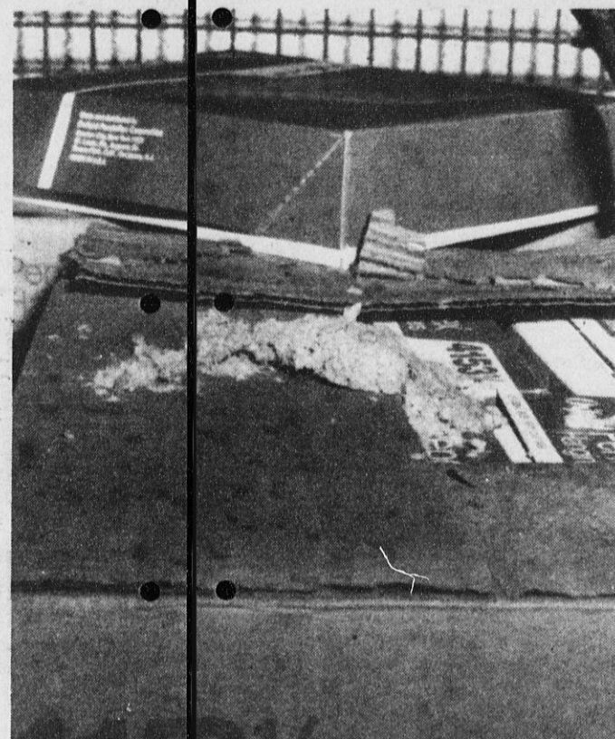
ASBESTOS, which had fallen from the ceiling of the warehouse at Bronx Psychiatric Center, sits atop a box. The material which clogs the ceiling contains cancer-causing asbestos, CSEA sources reported. Forty-eight operational employees are x-rayed and counseled because of long-time exposure to the deadly substance.
