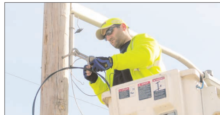
Town of Hempstead street lighting crew member Nick Acuri repairs a streetlight in North Valley Stream, a hamlet within the town.
