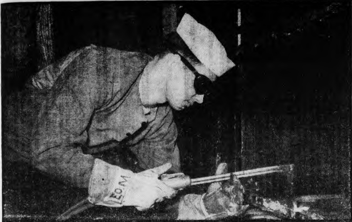
Here's a shipfitter using an oxy-acetylene torch. Both in Navy and in civilian life, the need for shipfitters is great. The demand for welders continues heavy.
