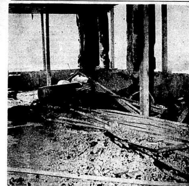
A PICTURE OF DESTRUCTION depicts the aftermath of the fire that swept the partially completed dormitory tower Thursday. The propane gas tanks amidst the rubble are blamed for the fire.
