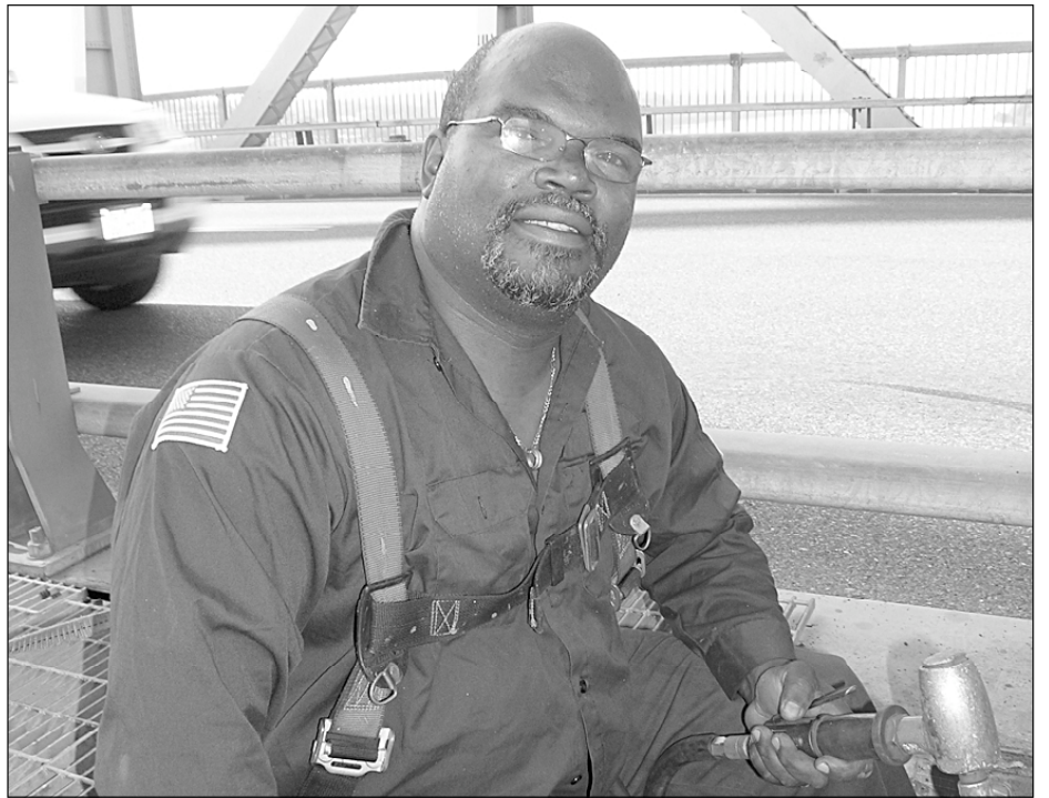
CSEA New York State Bridge Authority Local member David Hawkins works on bridge maintenance recently. CSEA members across the state perform similar work keeping New York’s bridges safe.
