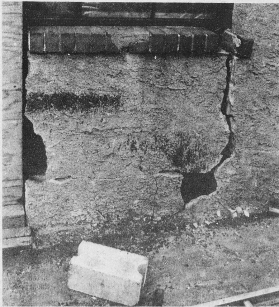
THIS SECTION OF THE OUTER STRUCTURE is unstable, could be easily moved by hand, and barely supports the window.
