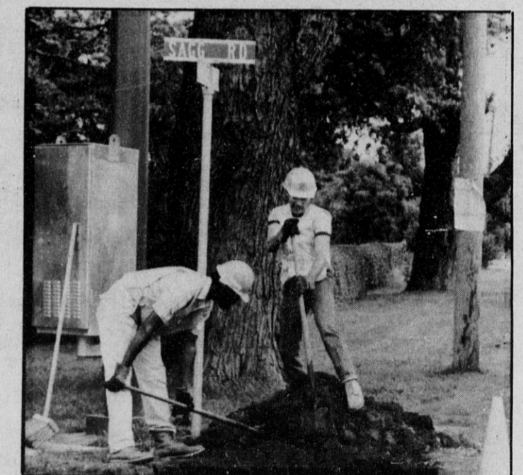
CSEA DOT LOCAL 508 members Richard Lewis, left, and Tom Burchell work on a highway in Hampton Bays.
