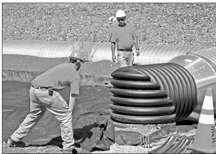
Delaware County Department of Public Works employees Ryan Boice, left, and Jerry Ford, right, work on landscaping outside pipes that carry air from the compost facility and filter it through the pile of cedar chips behind them.
