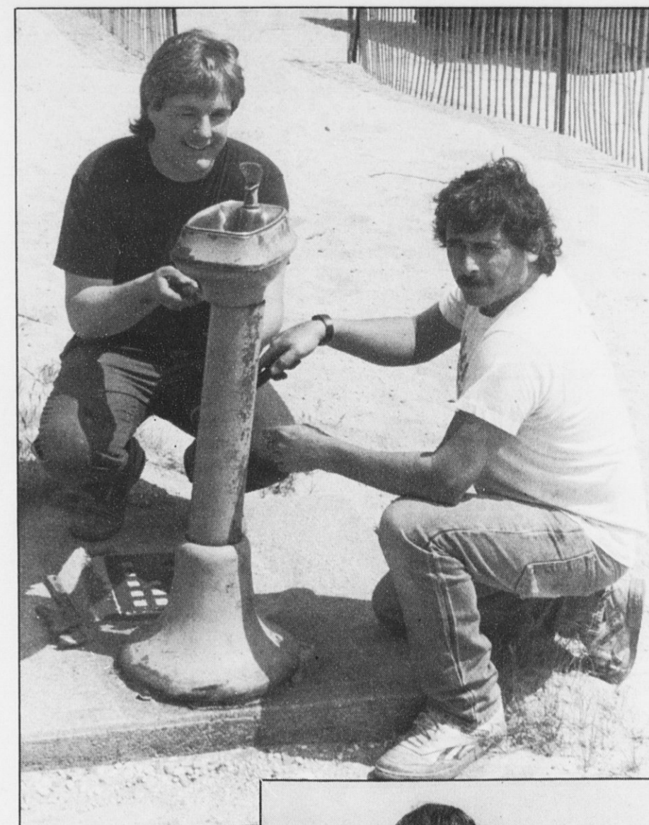
PLUMBERS Jay Skidmore, left, and Guy Knoblauch helped repair hundreds of water fountains and pipes at the parks all winter.
