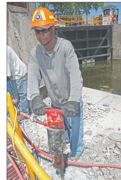
Laborer Mike McFadden uses a jackhammer to chip away concrete around the stairs at Lock 24 in Baldwinsville, where he and his co-workers are working to rebuild the stairway.
