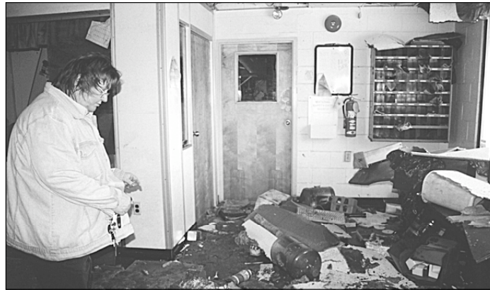
Port Jervis School District Unit President Betty Lou Kranz observes the damage floods did to the district's transportation garage.
