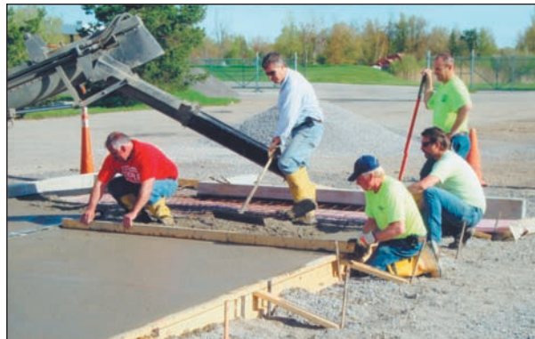
Members of the CSEA Clarence Blue Collar Unit, from left, Joe Daigler, Dennis Raquet, Paul Engler, Ray Valentine, and Chip Moore, work on the foundation of the new Clarence Animal Control Shelter.
