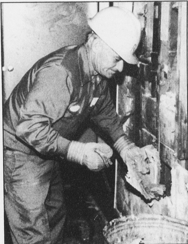
City worker Rossi Rotundo removes a portion of fire-damaged wall in the city court building in Middletown.
