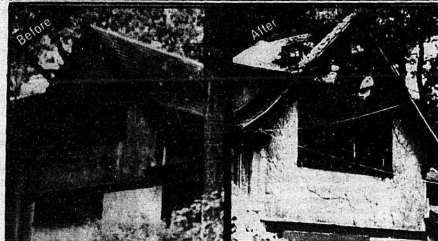
Chapel House before and after the fire. The basic structure is still intact.
