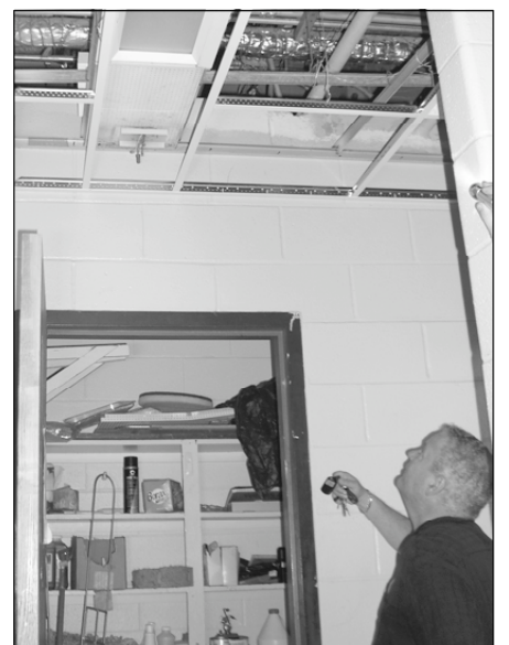
CSEA Labor Relations Specialist Jim Wall examines the site of an electrical accident that killed Michael Sallee at Miller Place High School in this file photo from 2005.
