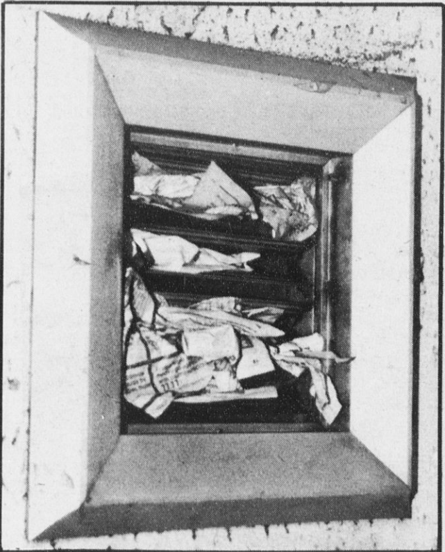
POOR VENTILATION means occasional bouts with sickening fumes and open fire doors as workers try to fight stale air in the dreary building. This ceiling vent, stuffed with newspapers, contributes to the problem.
