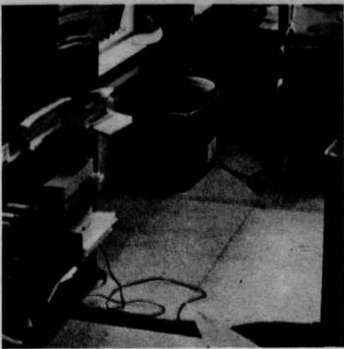
The Department of Labor's WIN program office in Buffalo is the cause of many complaints about working conditions. Electrical cords form one hazard.
