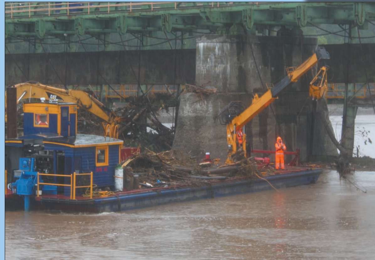
Above, state Department of Transportation workers, represented by CSEA Black River Valley State Employees, Clinton County State Transportation, Franklin County State Transportation, and St. Lawrence County State Transportation Locals, work to fix a collapsed roadway in Elizabethtown, in Essex County.
