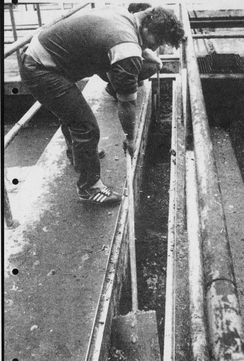
THE FACILITIES MAY HAVE COST in excess of $100 million, but a design error requires Shop Steward Jim Abbatiello to use an old-fashioned paddle to move grease.
