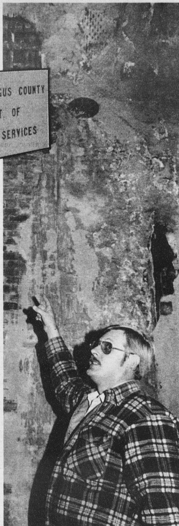
HALLWAY HAZARD — Local 805 President Robert Painter points out the condition of the back hallway that leads to the rest rooms.
