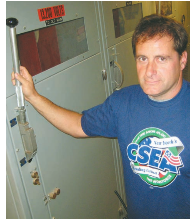
Fred A. DeStefano, an electrician, shows how he rushed to shut down electrical systems in van den Berg Hall at SUNY New Paltz in order to prevent a fire.
