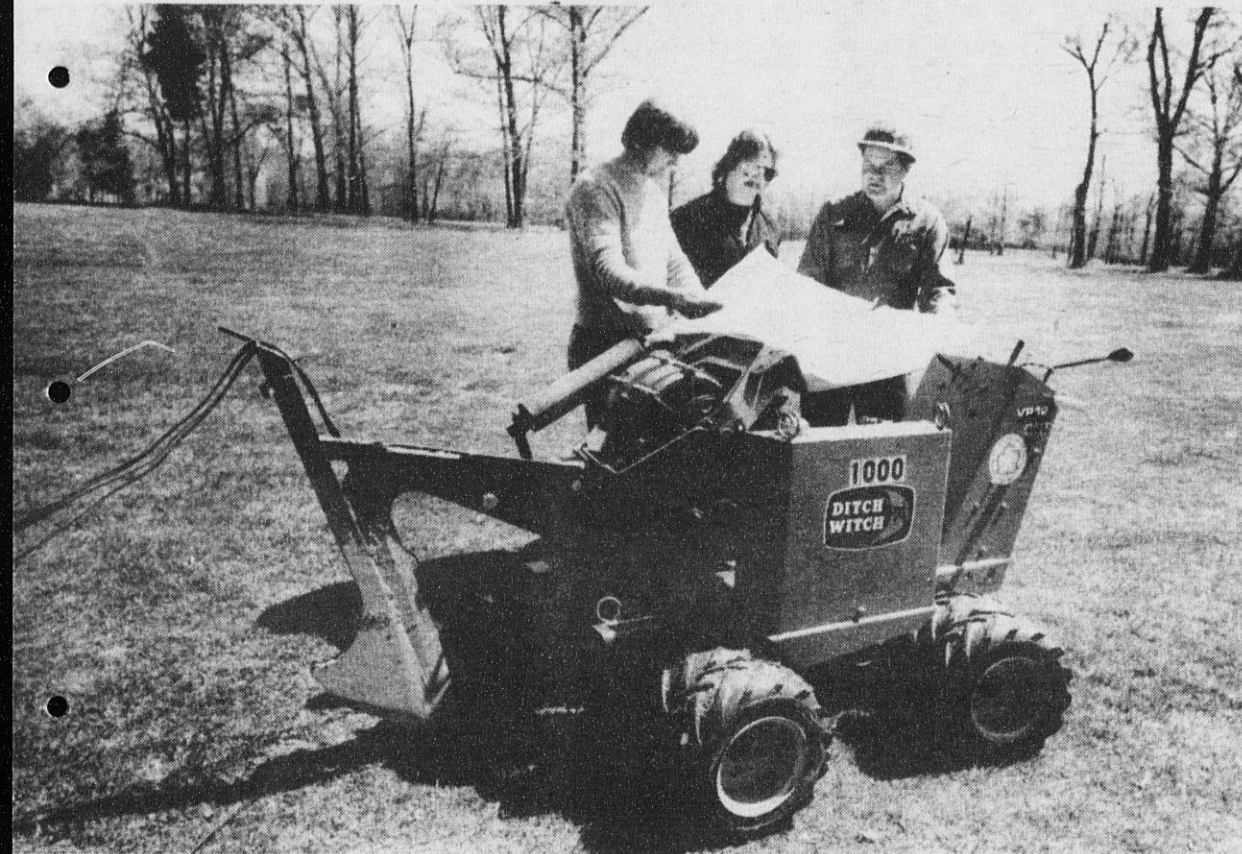
DITCH WITCH machine proved invaluable in installing the electrical system for the automated sprinkler facility. Electricians Supervisor Ray Dobbins, left, studies plans with electricians Pete Muscara, center, and George Walters.
