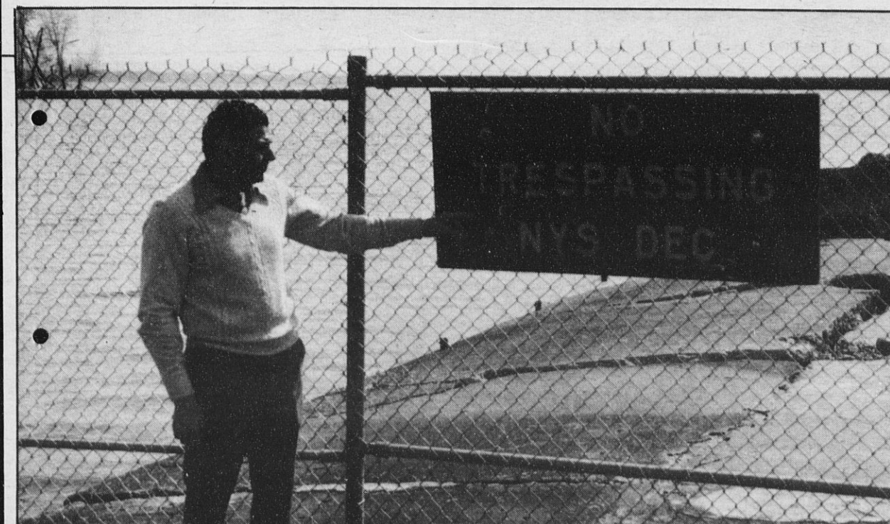
BARGE CANAL LOCAL 502 PRESIDENT Frank Zammiello Jr., a tireless fighter for the restoration of the canal to a useful waterway, points out the state's cursory effort to correct the breakwater problem with a fence and "no trespassing" sign.
