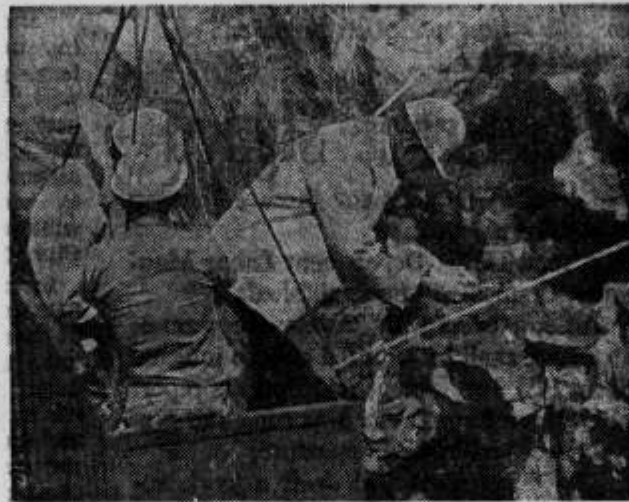
The three workers inch closer to the face of the gorge in their "man basket" to get a closer look at some of the rock.
