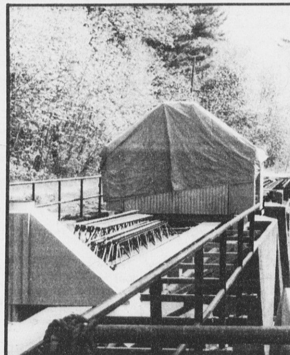
BOILERS which will be used in the incinerator process are covered by tarps while construction of the controversial system is progressing.
