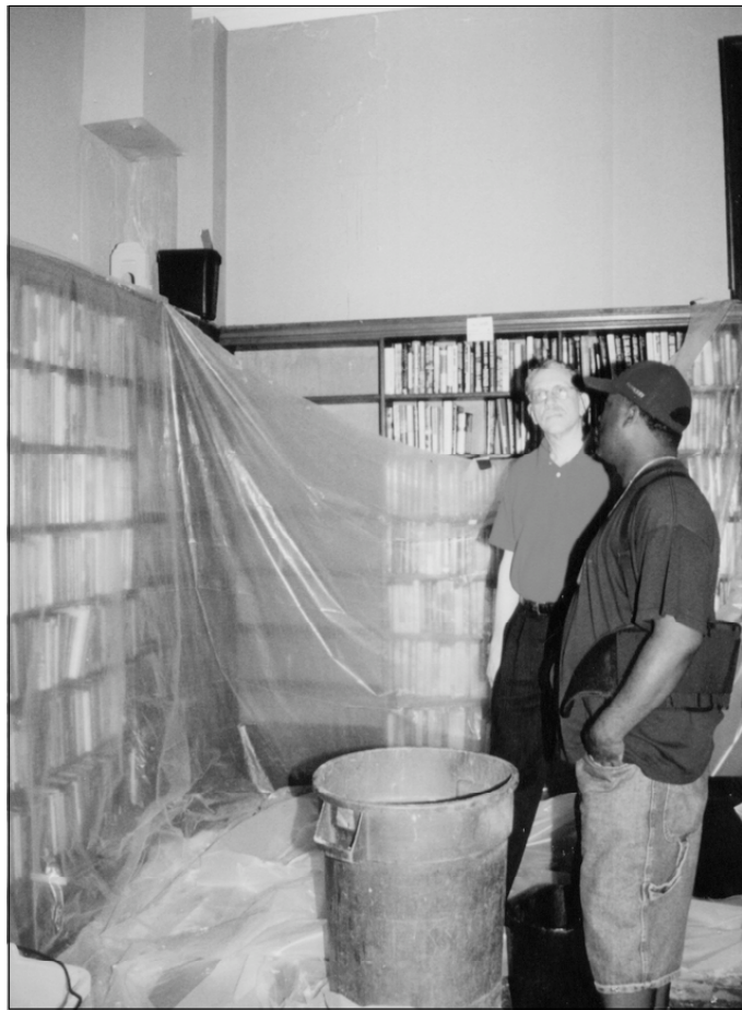
Mount Vernon Public Library Unit President Gary Newman, left, and 20-year CSEA member Jesse Vanlew, the library's head of maintenance, examine damage leaking water has done to a now-closed fiction room.
