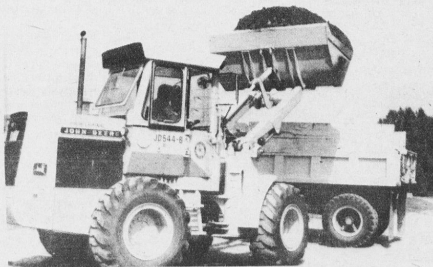
TOP SOIL from a site behind the campus is loaded on a dump truck for use elsewhere. Ed Nye is operating the loader.
