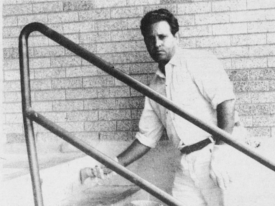
ANTHONY GUGLIUZZA paints exterior surfaces, a project done during the late summer and fall periods to afford protection against winter weather conditions.
