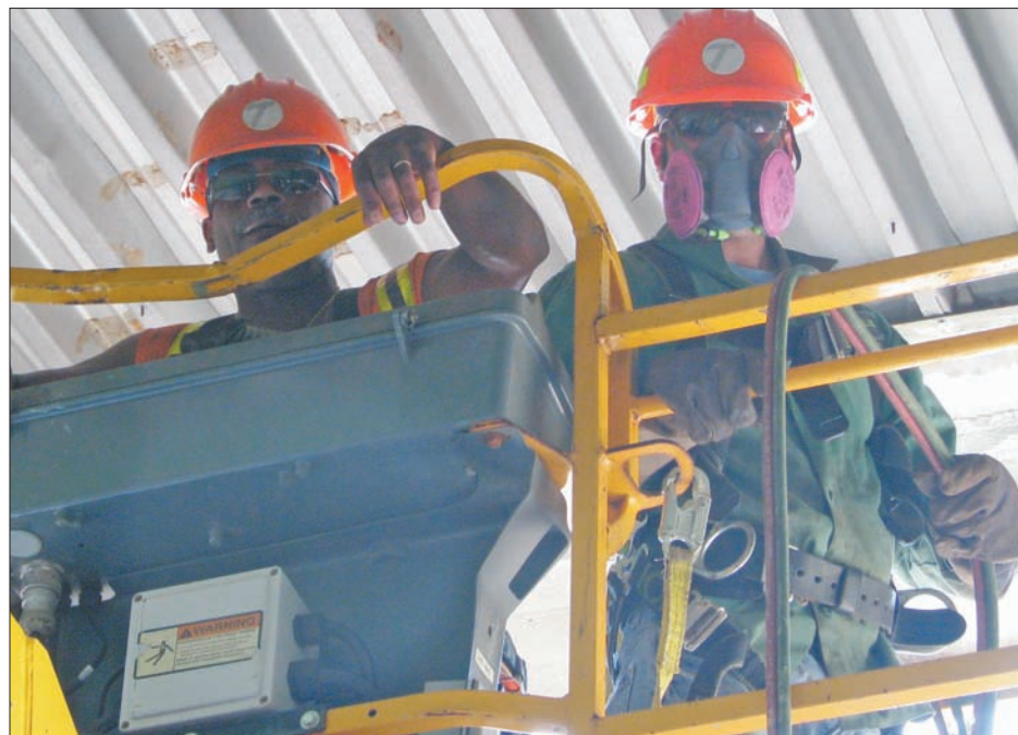
CSEA Long Island state Department of Transportation Local members Al Young (left) and Sam Ghabra make repairs to a Long Island Expressway overpass.
