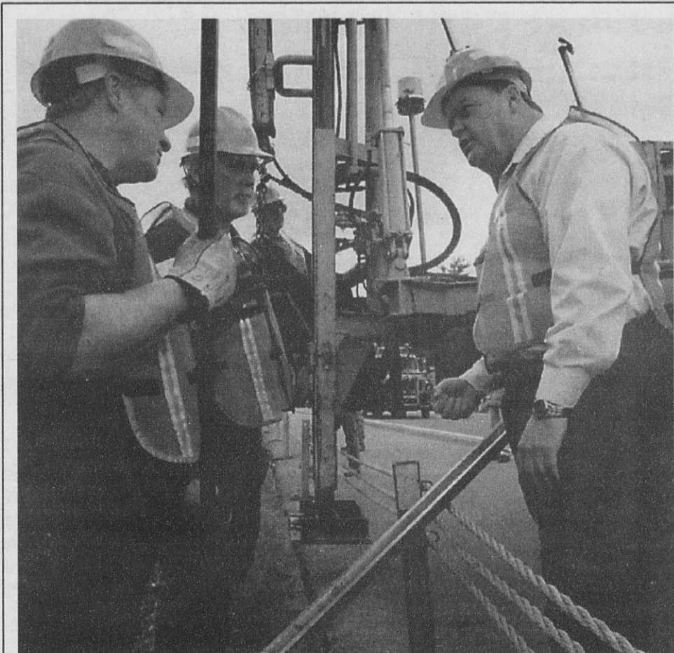
CSEA President Danny Donohue, right, hears safety concerns from state Department of Transportation workers Drew Thompson, left, and Peter Kolonsky, center, at an Adirondack Northway work site recently. The biggest concern for workers who maintain roads is speeders rushing past work zones. That's why the union has available bumper stickers with the message "Give 'em a brake." Call the Communications Department at 800-342-4146, ext. 1271, for a supply.
