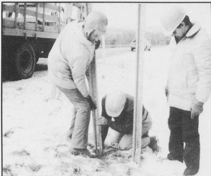
DOT WORKERS Walt Leight, Dick Pickering and George Ballard all say they wouldn't trade their jobs for another inside, even if they do need a jackhammer to bust up frozen ground during winter.
