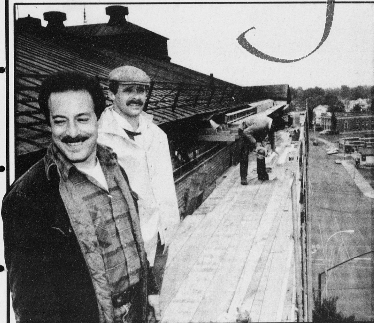
OVERLOOKING THE CITY OF SARATOGA SPRINGS from atop City Hall are CSEA Unit Treasurer Vince Arpey and Unit President Jim Brophy. Unit members in background are busy restoring the facade of the municipal building.
