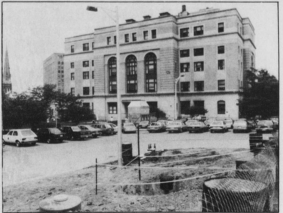
THE ONEIDA COUNTY COURTHOUSE was the site of a recent explosion and fire blamed in part on a major gasoline leak in the soil. In the foreground is where the county replaced gasoline storage tanks.
