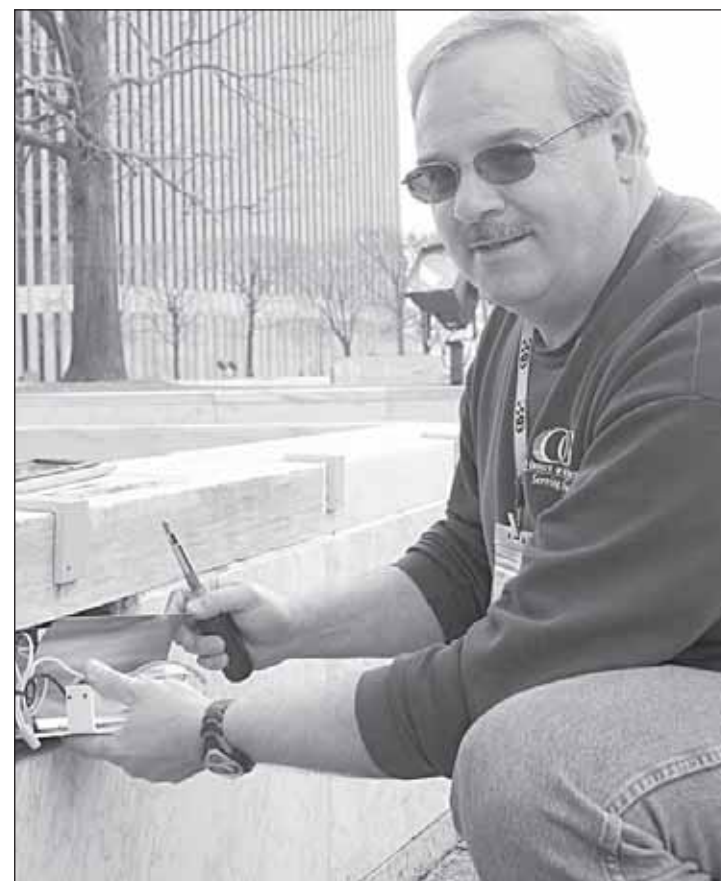
State Office of General Services electrician Frank Salvagio installs an improved light fixture he designed into a marble wall at the Empire State Plaza.
