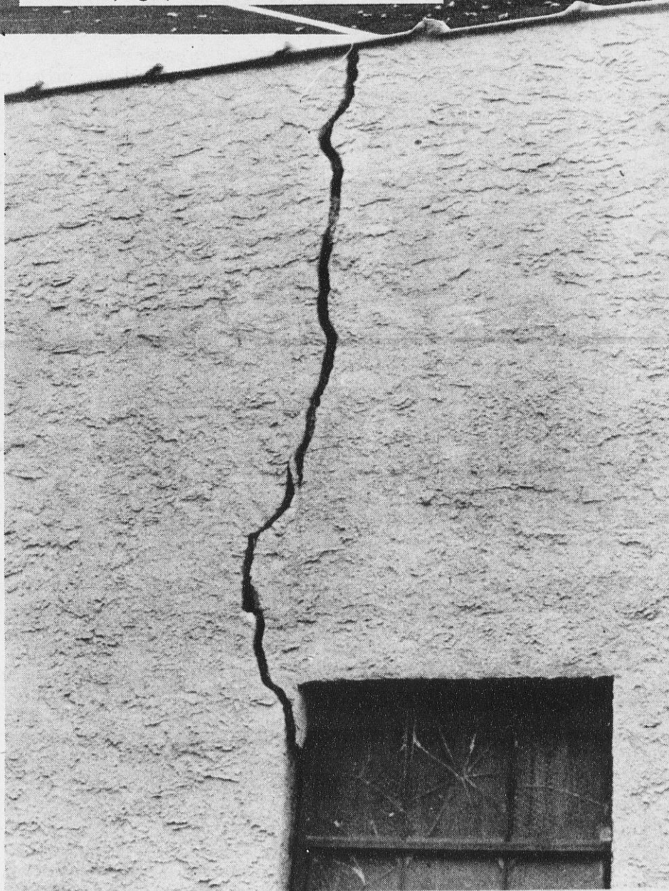
NEW NORTH TARRYTOWN GARAGE, above, is far cry from the former village garage where cracked walls, below, and deplorable working conditions, right, were commonplace.
