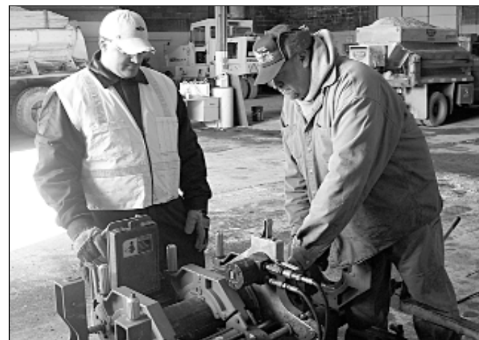
Colonie Unit B members James Hildenbrandt, left, and Bill Alund fuse pipes to create the network of gas pipes under the Colonie landfill.
