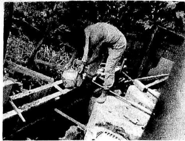
IN SHARP CONTRAST to Japan's widespread technology, a worker carries cement in buckets for a modern sewer.
