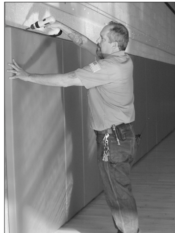
Levittown School District member Scott Torrance fixes the padding in the gym.
