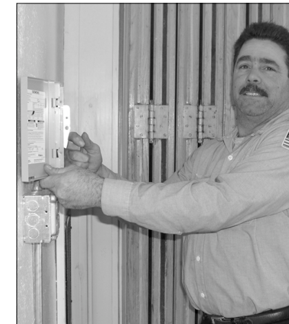
Levittown Electrician Joe Carbonaro checks the power source for the remote bleachers in the gym.
