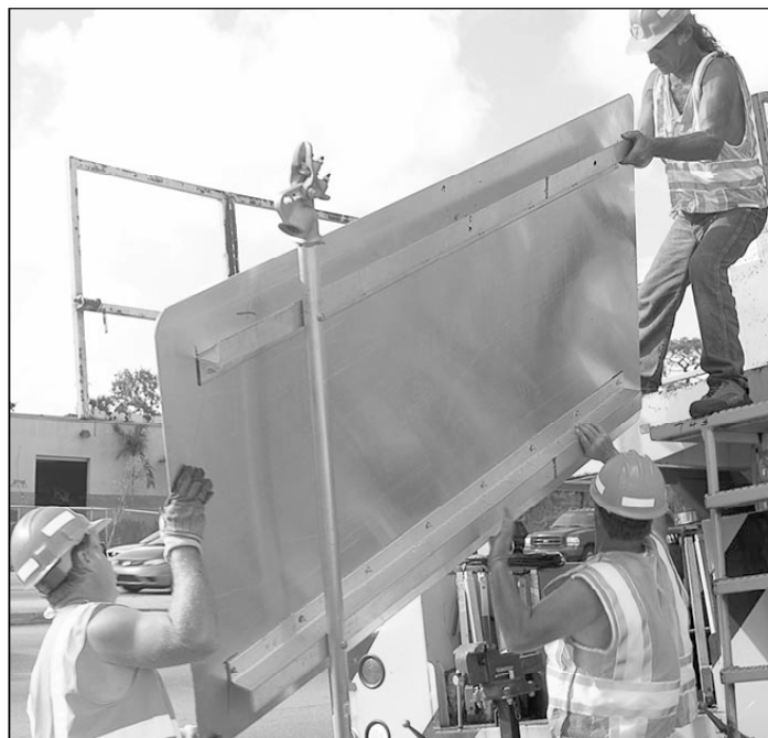
State DOT workers load a road sign in preparation of replacing one damaged by Hurricane Wilma.
