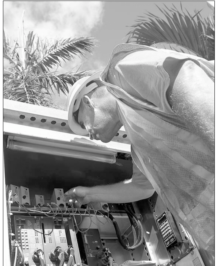
A state DOT worker from Utica helps repair traffic signals in Broward County, Florida. Workers were called in to help in the wake of Hurricane Wilma.
